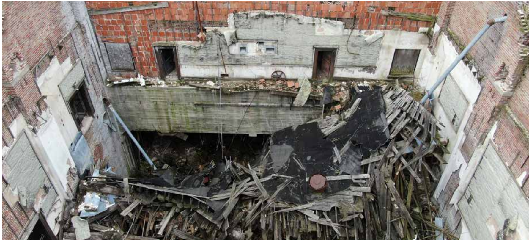
COLLAPSED ROOF OVER THEATER AUDITORIUM
