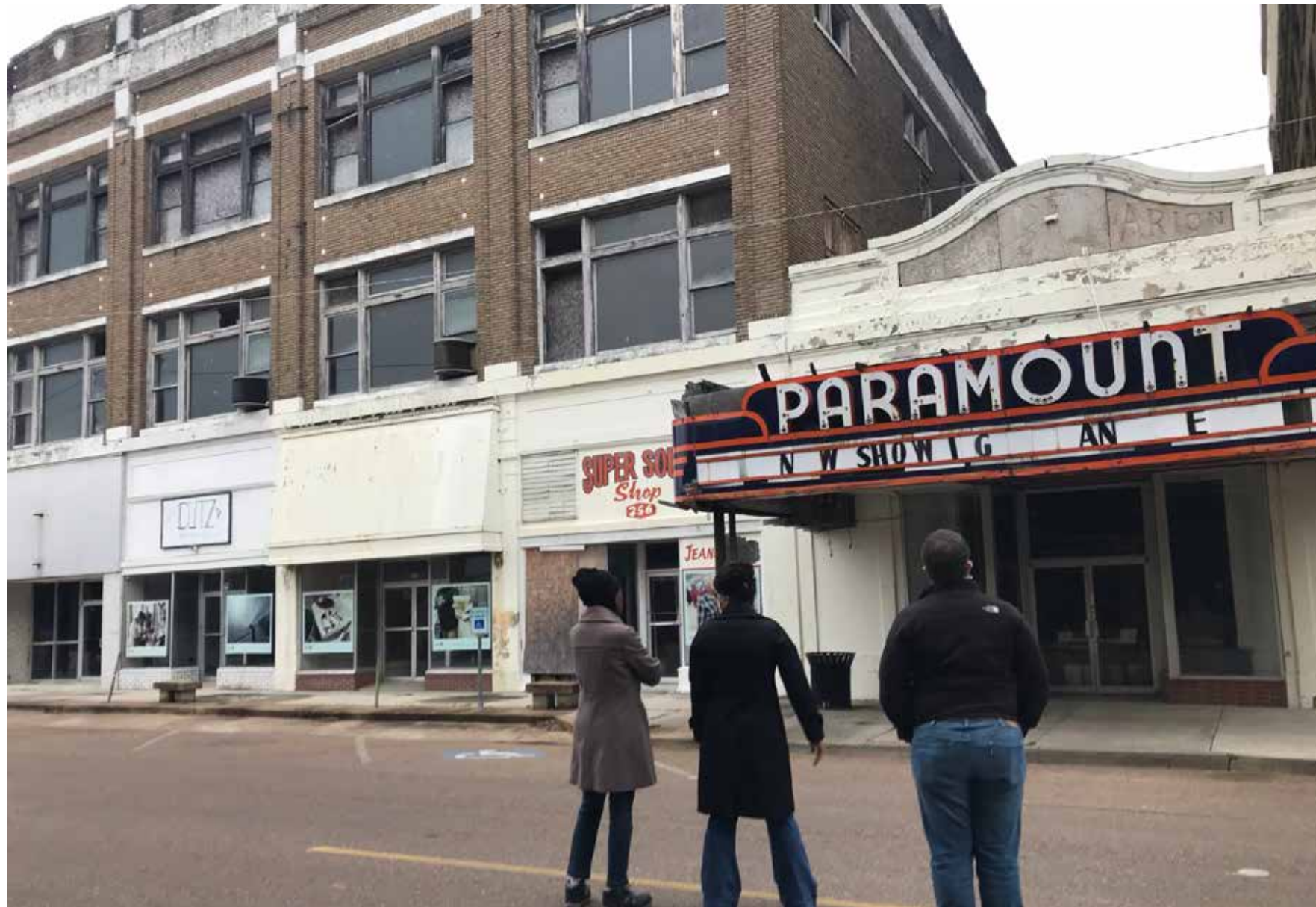
CURRENT CONDITION OF ICONIC PARAMOUNT THEATER MARQUEE, WITH ADJACENT DEPARTMENT STORE WINDOWS IN DISREPAIR
